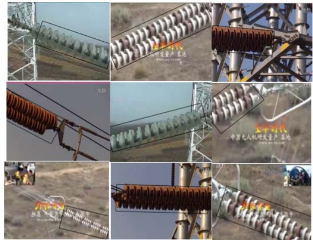
Fig. 10: The insulator detection
