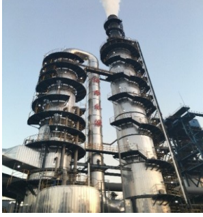
Fig.1 Desulfurization and denitration integrated device for coking flue gas
